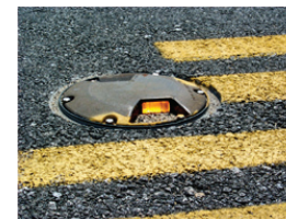
In-Pavement Runway Guard Light
